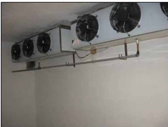
Cold Storage Room
